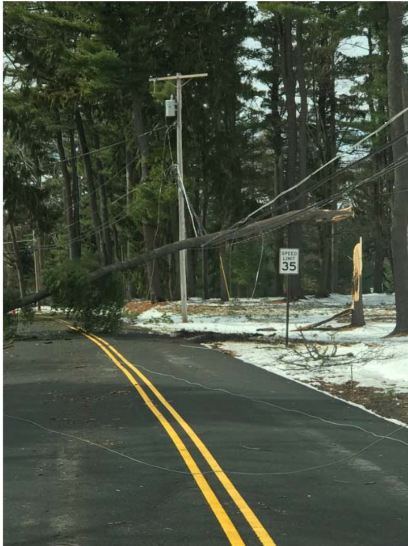
March Winter Storm Damage in Summit
